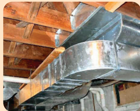
Proper air duct maintenance helps ensure cleaner indoor air for your home.
